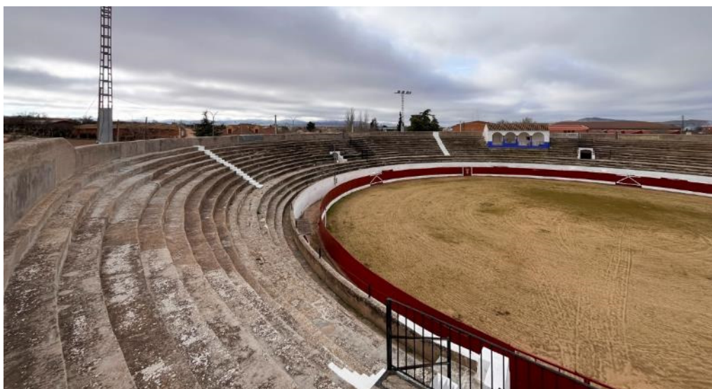
Vista general tendido sureste (sol)
